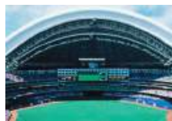
Roof of the Skydome in Toronto, Canada (parabola) Walter Schmid/The Image Bank/Getty Images
